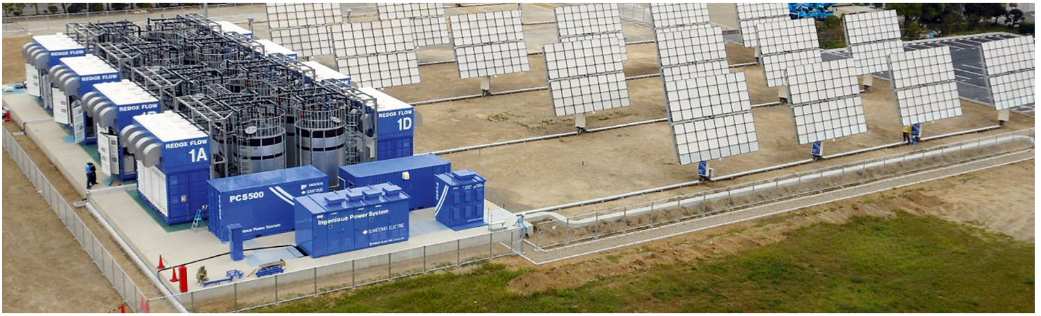
Sumitomo Electric, Yokohama Works, 1MW-5MWh, this application provides for demand side management, renewable Integration and renewable firming.
