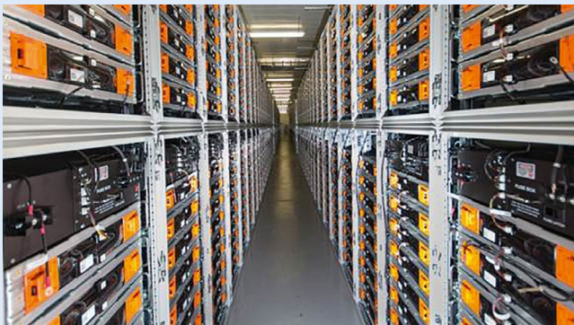
Southern California Edison Tehachapi Wind Energy Storage Project
